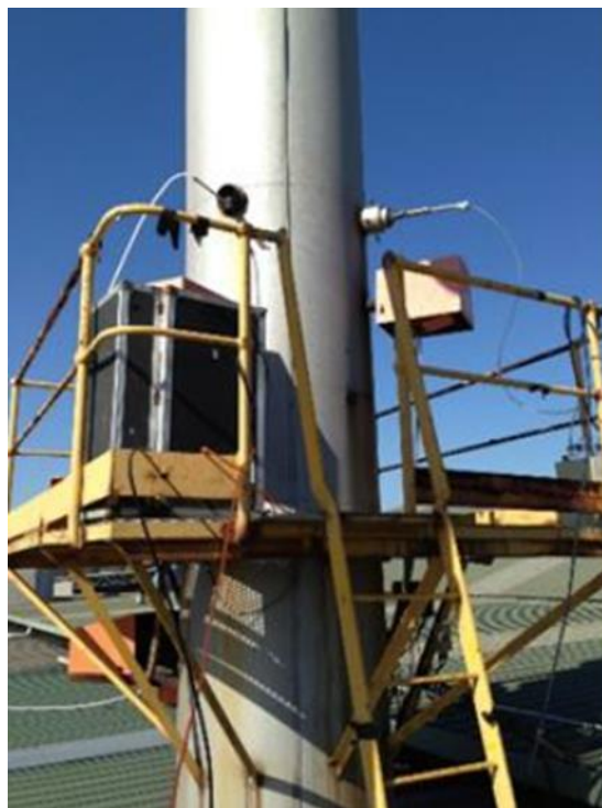
Image 1. EPA 1 – Afterburner Discharge Stack
