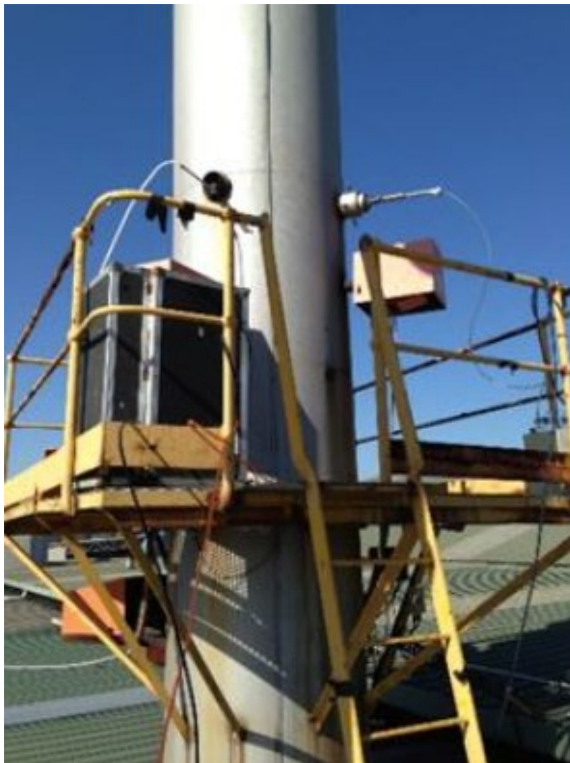
EPA 1 – Afterburner Discharge Stack
