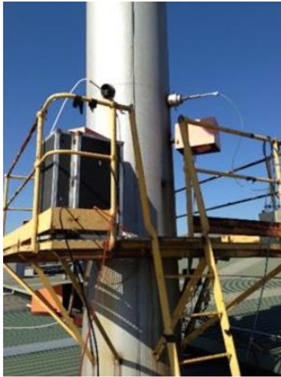
EPA 1 – Afterburner Discharge Stack
